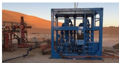
HP solids removal systems.
