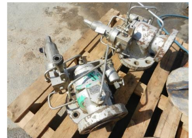
Pressure Safety Valve re-calibration.
