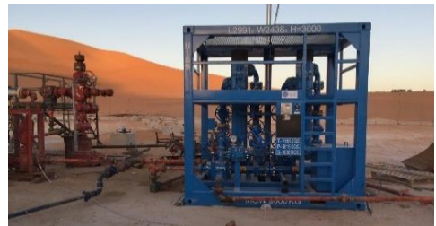
HP solids removal systems.
