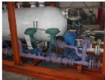
Separator, SAS, BOP, etc...
